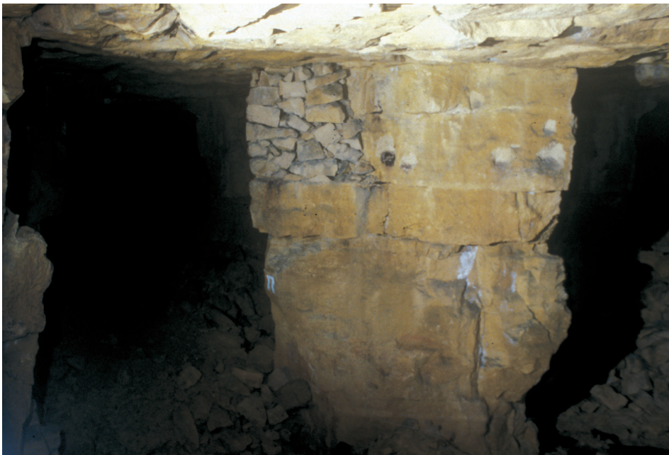
Fig. 8.15 Stone used to pack up the top of a pillar where it had been intruded upon by the picking bed, east Firs
