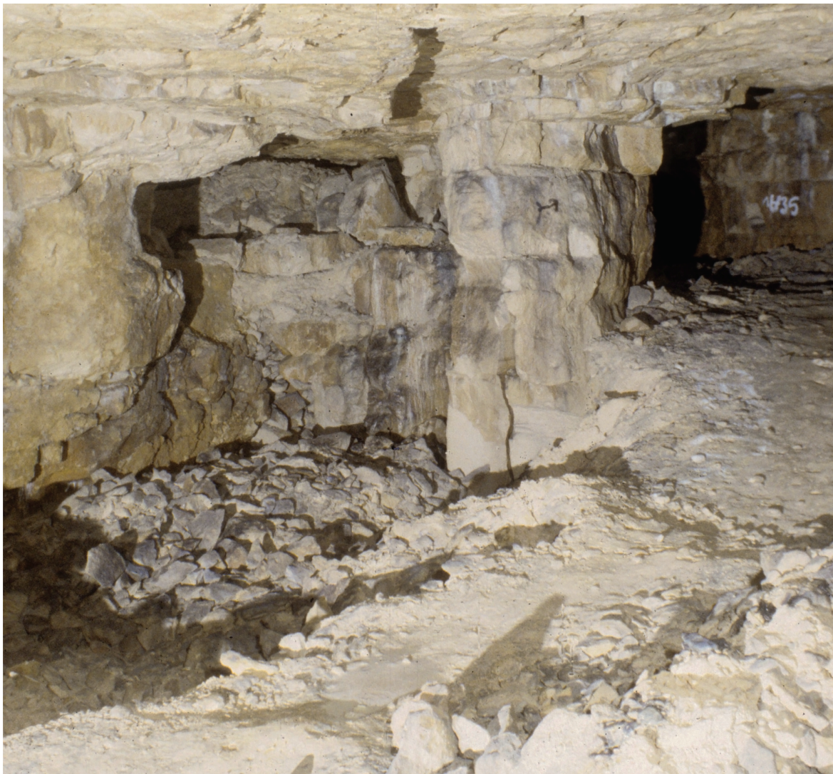
Fig. 8.1 Remains of a picking bed entry at top centre, about 0.9 m high in East Firs (Quarry 2205)
