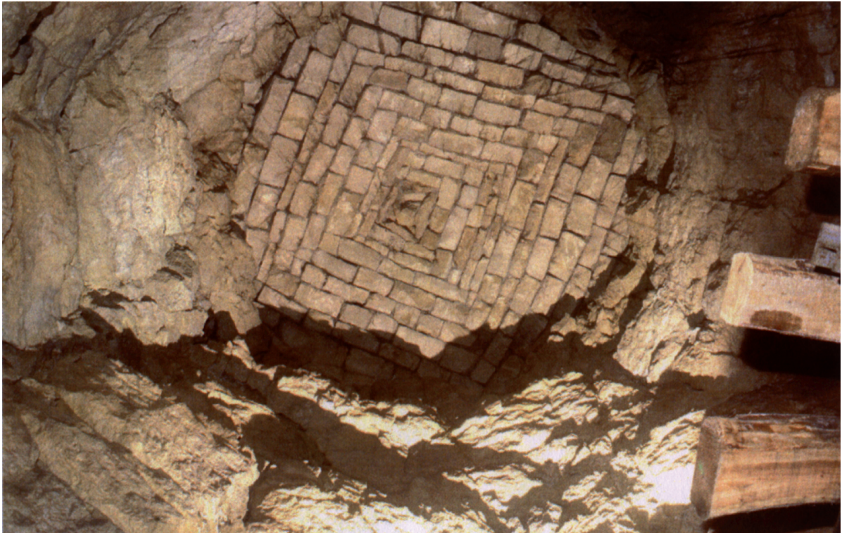
Fig. 9.9 Shaft cap above cartway (2194) viewed from the underside, associated with Allen Phase II workings in East Firs (Quarry 2206)
