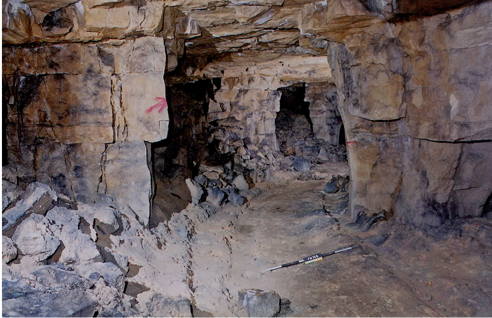
Fig. 9.13 Nineteenth-century cartway in East Byfield, showing rub marks caused by a cable on the right side pillar, and wheel ruts on the floor
