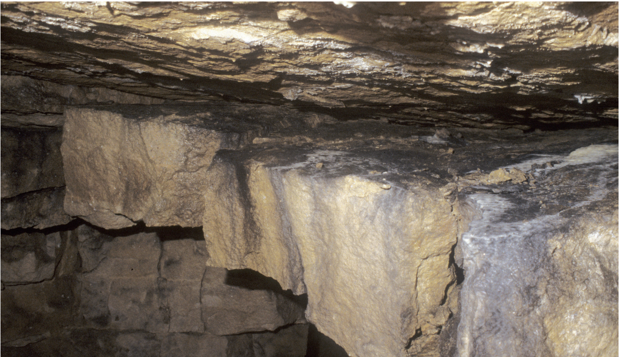
Fig. 10.15 Delaminating roof bed in Central Firs (Quarry 2211)
