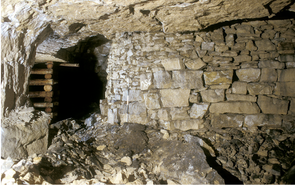
Fig. 10.29 Bathite blocks used to support roof under the rear of the Hadley Arms
