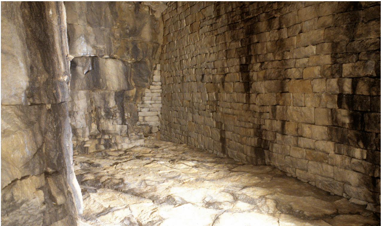
Fig. 10.12 Substantial rubble and blocks used to construct the wall near the Hadley Arms under the south side of North Road
