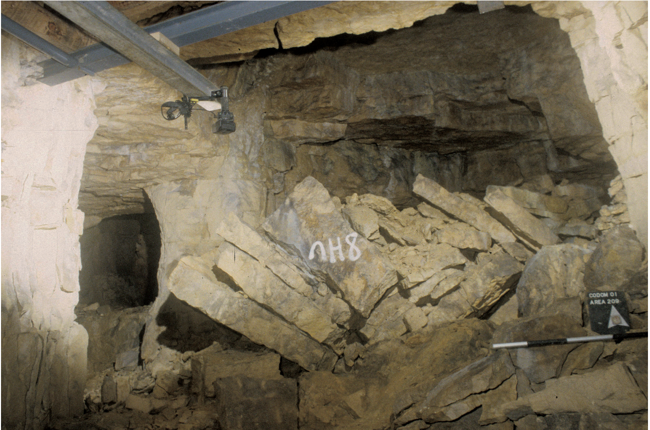
Fig. 10.16 Collapse of Twinhoe Beds in East Firs
