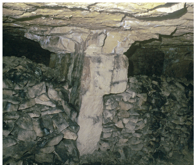
Fig. 10.8 Corbelled pillar just west of Firs Shaft, with inadequate support in the core width below
