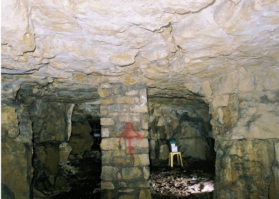
Fig. 10.13 Rubble stone mortared packs under a municipal drain running across the surface overhead in West Byfield
