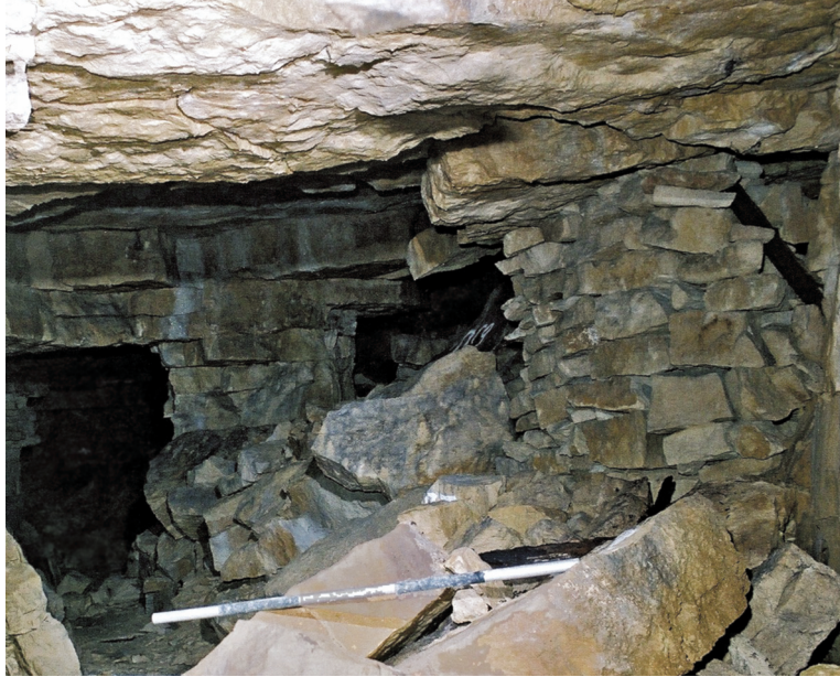
Fig. 10.18 Pack built on top of fallen blocks in Central Firs (Quarry 2200)
