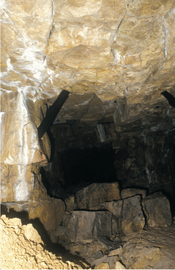
Fig. 10.14 Fallen blocks in Byfield (Quarry 509)
