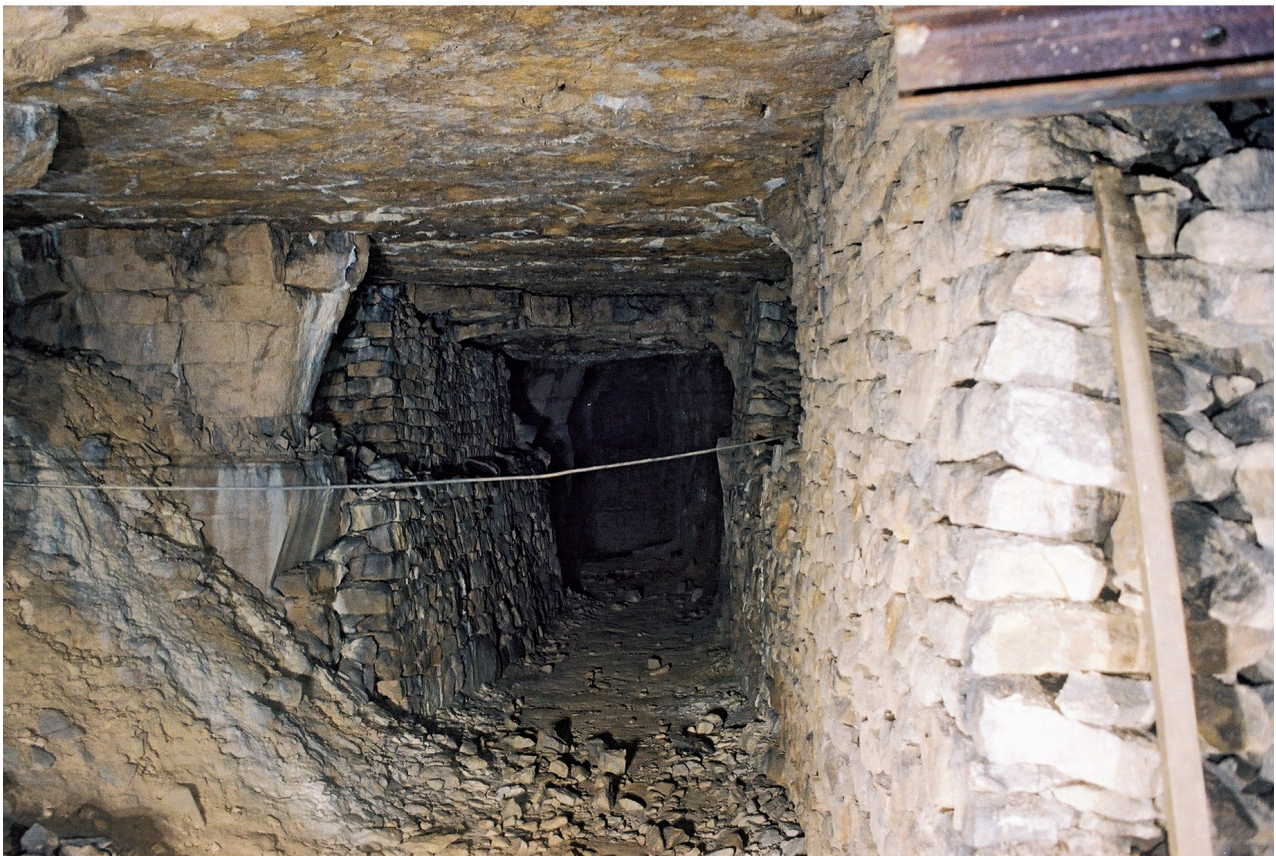
Fig. 10.27 Flanking roof support packs in the first section of Allen's west cartway from Sheeps House Quarry
