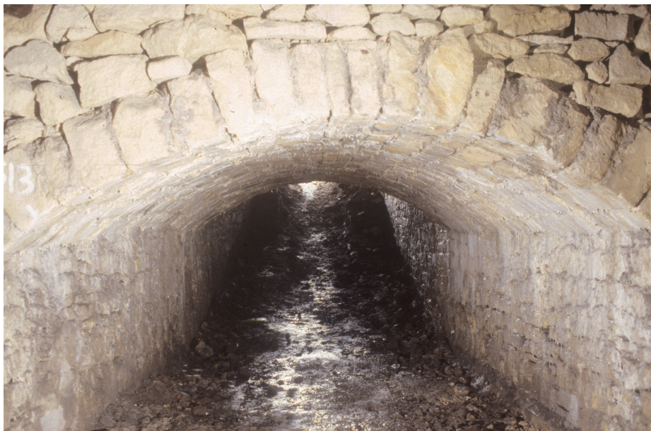
Fig. 11.6 The Irvings Incline, a slope entry into the West Byfield, Hulonce Quarry (504) made early in the 19th century and variously used for storage and an air-raid shelter after quarrying finished
