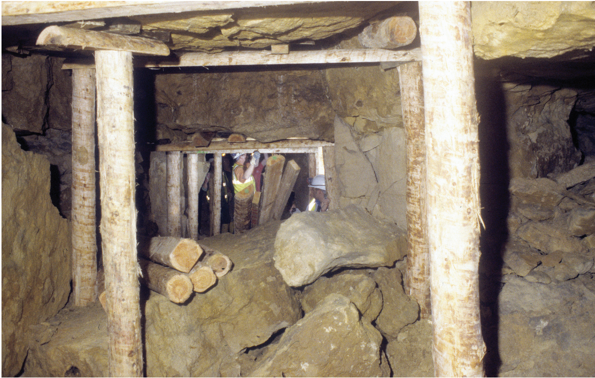
Fig. 12.23 The unstable lower working in Scrace's quarry (Quarry Area 512, Byfield)
