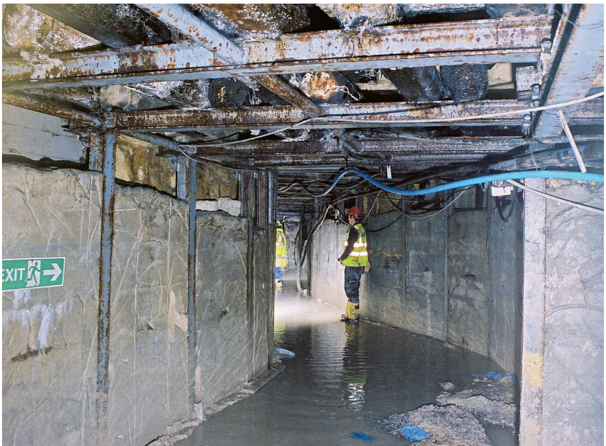
Fig. 1.7 Steel supported section of Roadway 2 in east Firs, after concrete had been emplaced
