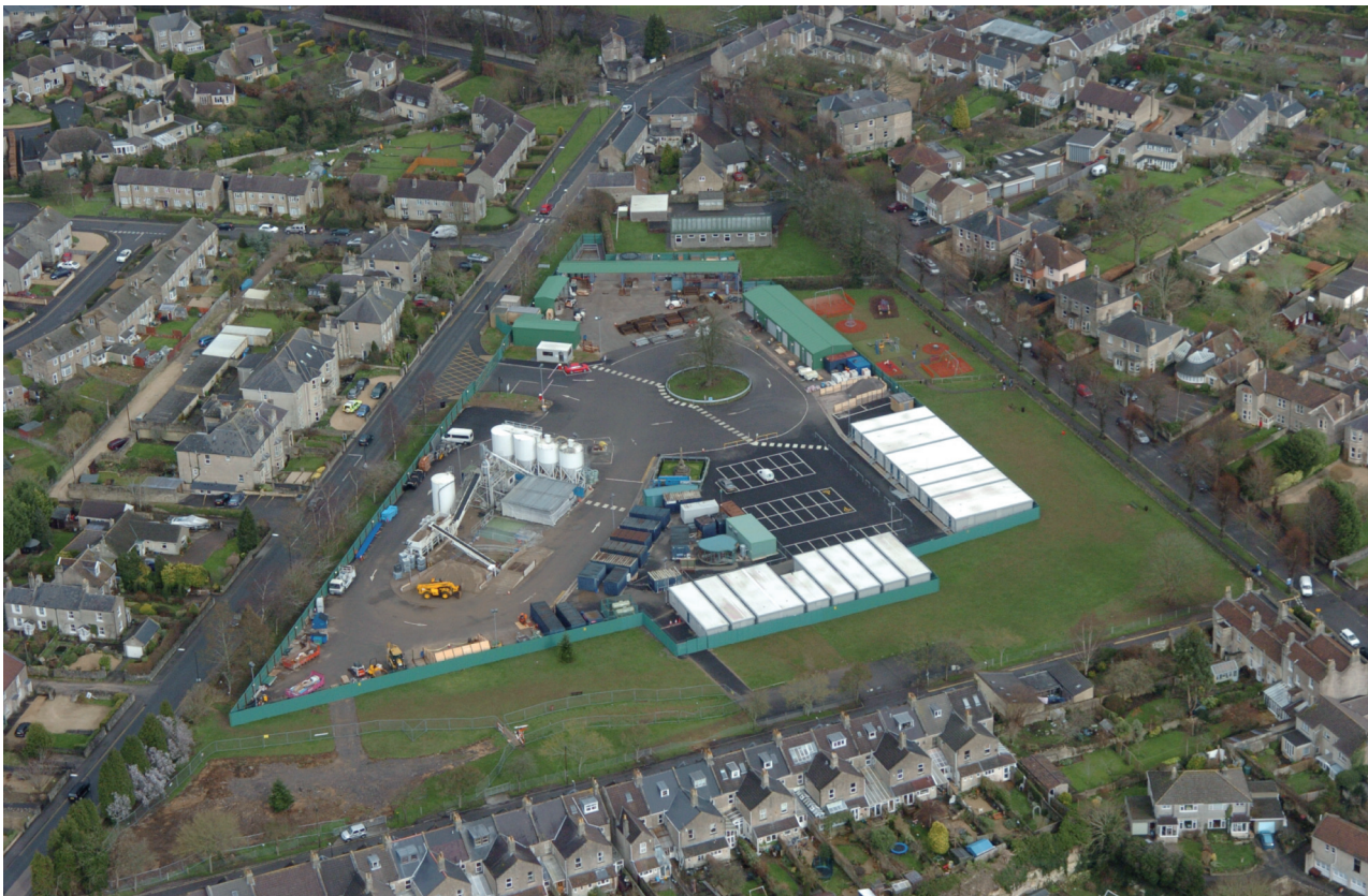
Fig. 1.4 Firs Field during the stabilisation project, view east. Firs Shaft is covered by the green circular roof in the centre foreground, and the Materials Shaft (the former Arched Shaft) is at the right of the long green-roofed building in the background (Image courtesy of Bath & North East Somerset Council)
