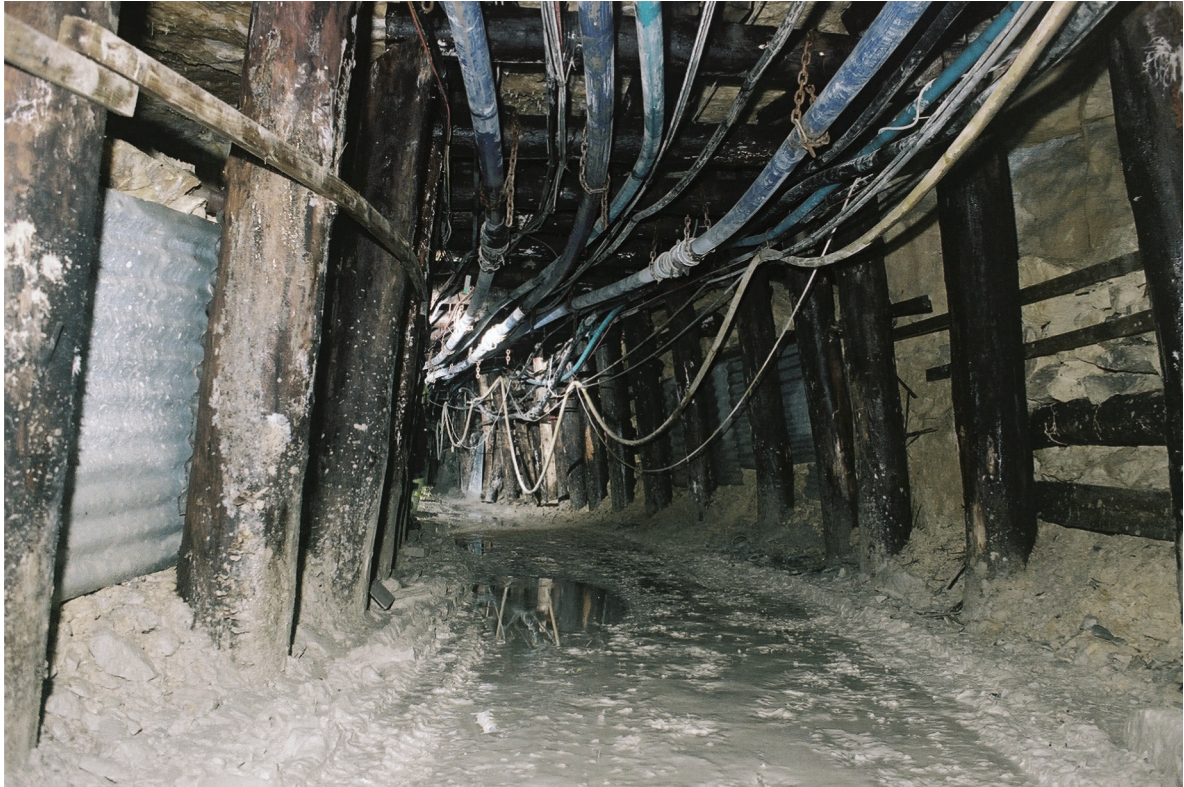
Fig. 1.6 Timbered support on modern roadway 2 near Firs Shaft. The blue pipes delivered the concrete used for infilling
