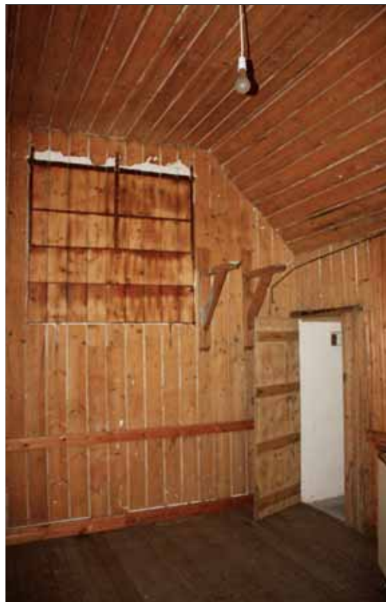
Plate 24: Evidence of removed cupboards and internal door, G4
