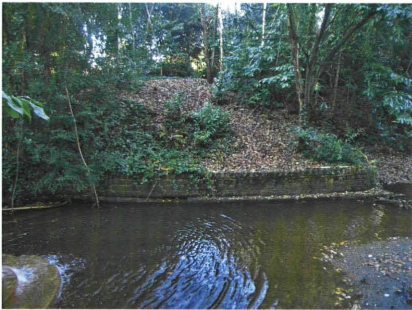
Plate 2: West wall of Southern inlet, showing subsidence
