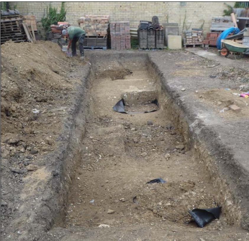
Plate 2: View of Trench 1 with Terram laid over the exposed burials prior to backfilling of graves by hand, taken from south
