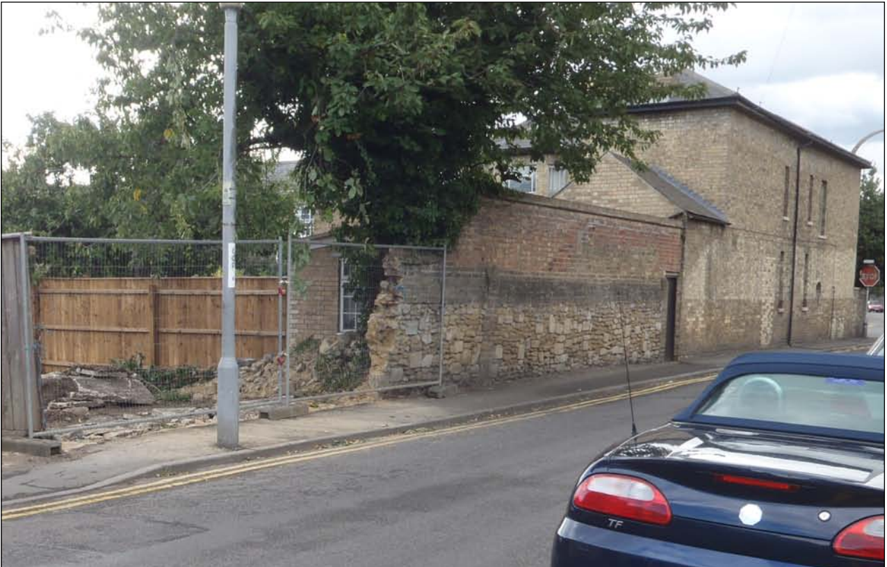
Plate 1: View of stone wall on south side of Victoria Street, taken from north-east
