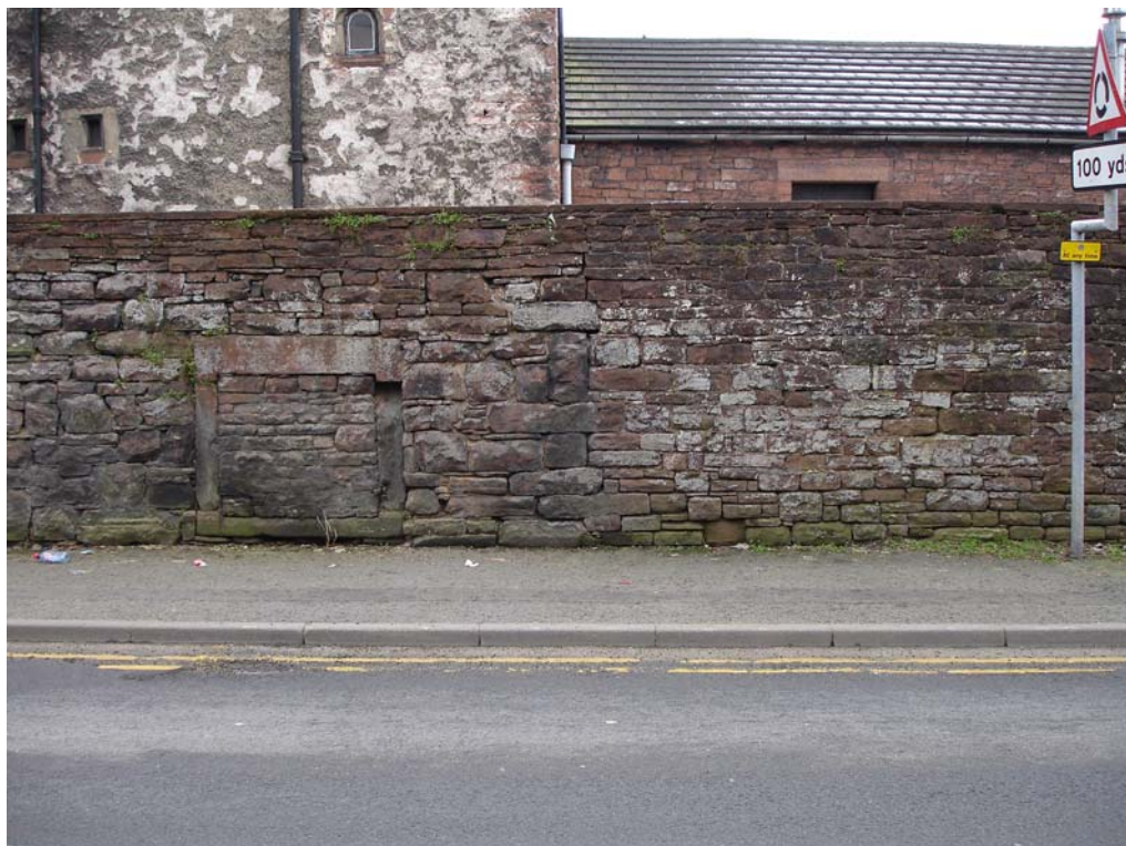
Plate 5: Third aperture and possible vertical join in the wall forming the site boundary along Benson Row
