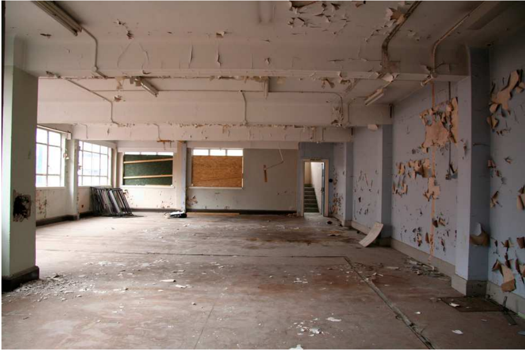
Plate 25: Third floor stripped-out open plan office with floor scars showing locations of demolished partition walls 17
