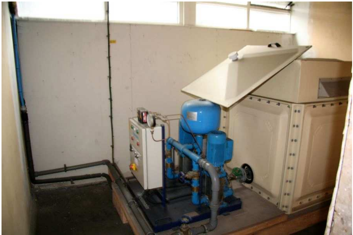
Plate 53: Waterpump and tank
