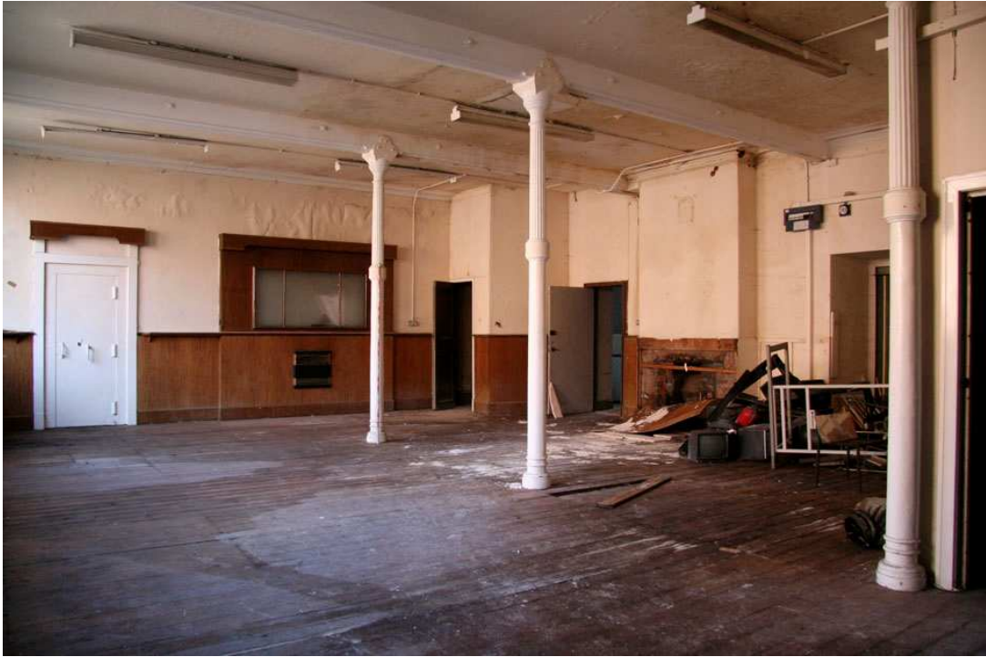
Plate 7: Ground floor open plan office 2 showing the column arrangement and strong room set into the east wall
