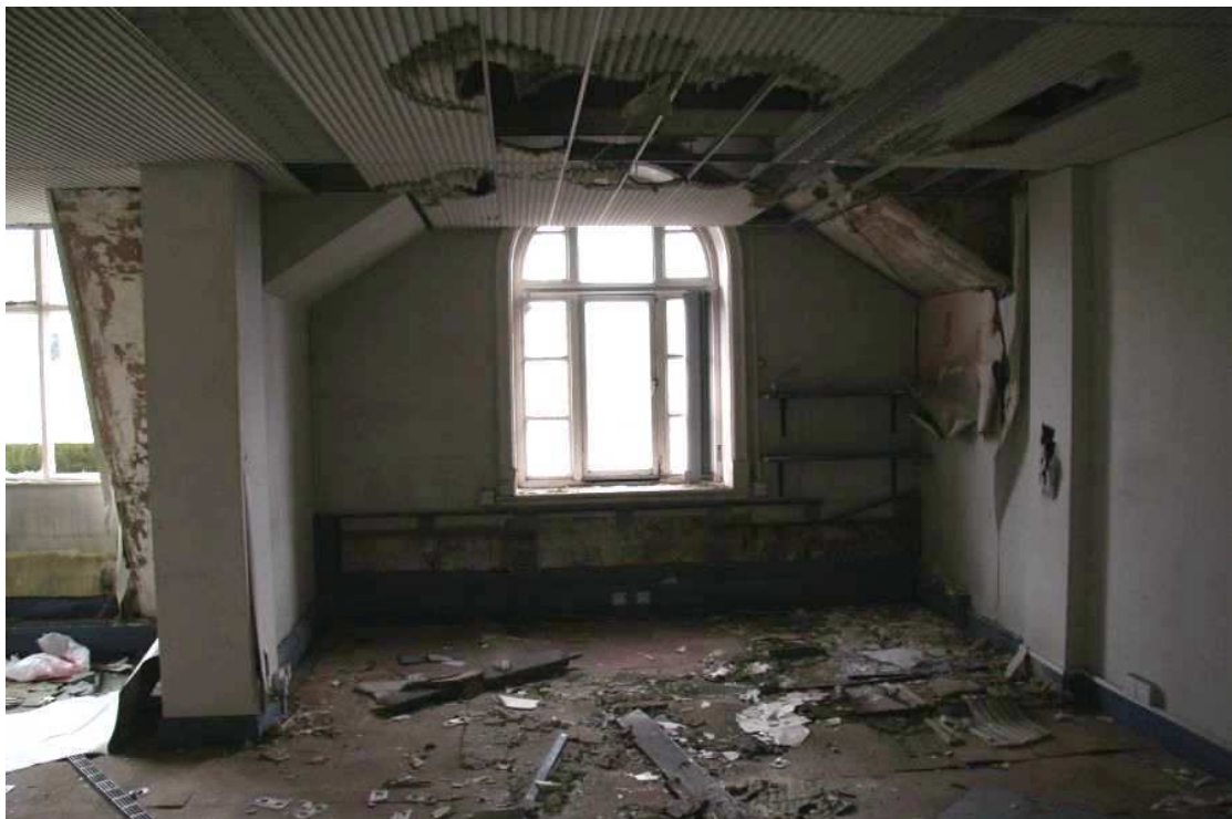
Plate 64: Central arched window beneath broken pediment on the fourth floor, showing truncation by the suspended ceiling
