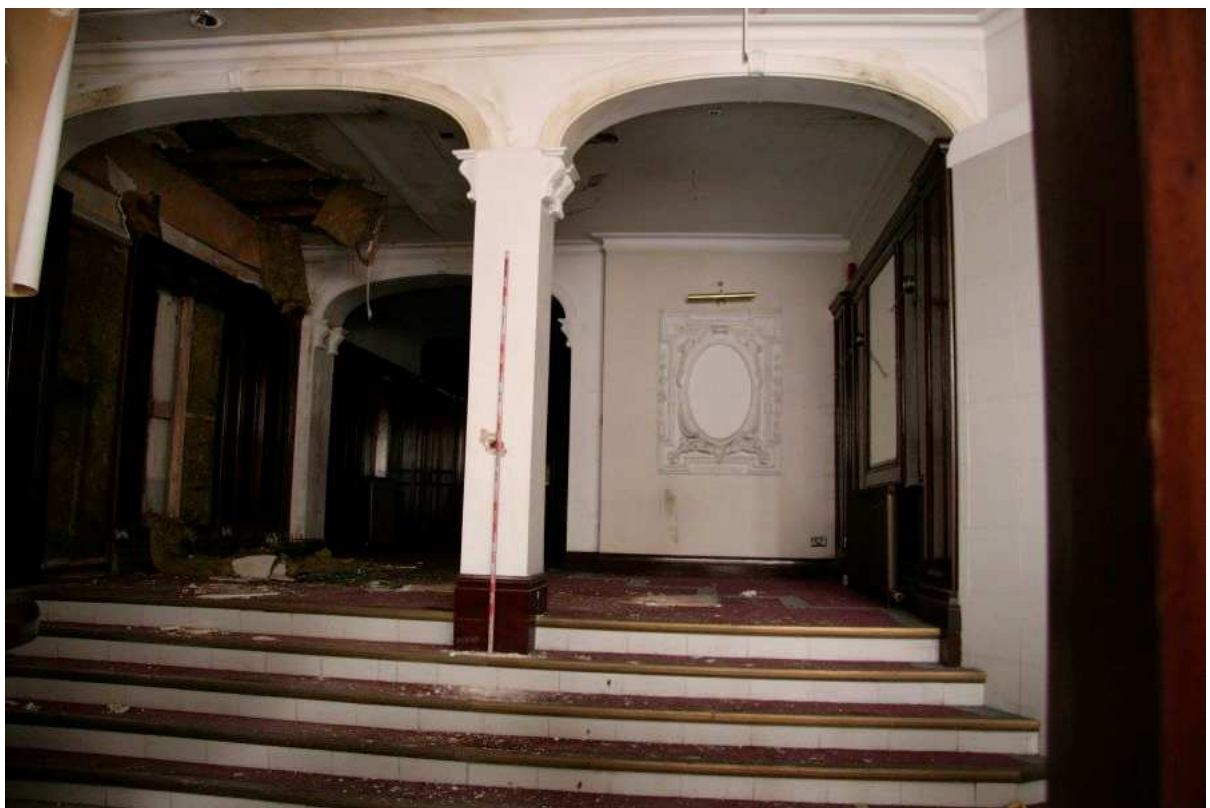
Plate 56: Foyer and main entrance at the south side of 67 Dale Street showing off-the-peg plaster mouldings
