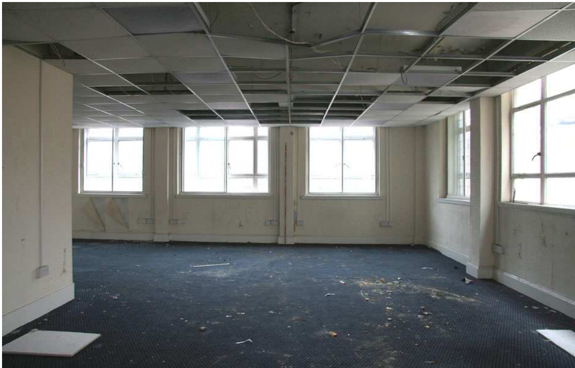
Plate 26: Third floor open office 17C showing suspended ceiling obscuring full height of original windows, plus column arrangement in south and west facing side of structure
