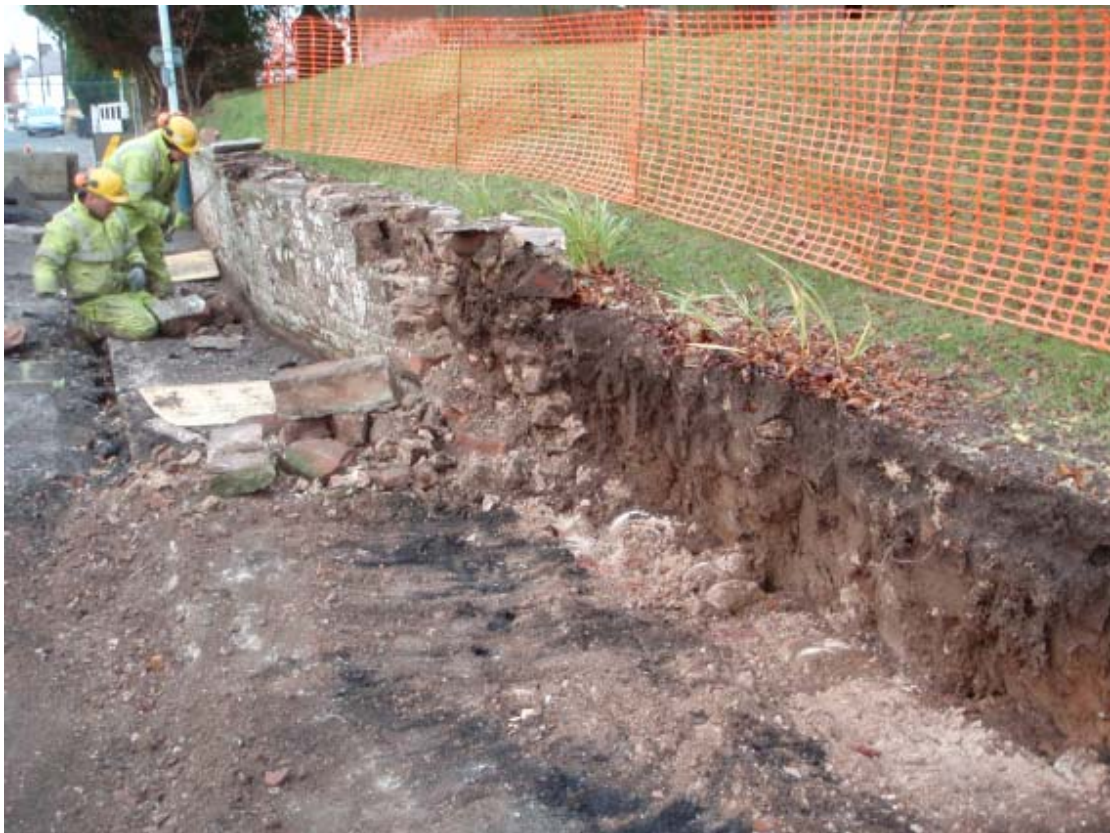
Plate 4: Working shot of the removal of the church wall and the revealed churchyard deposits
