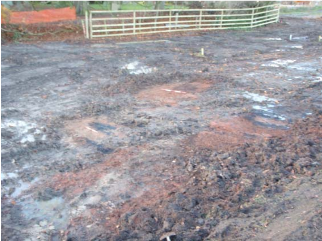
Plate 1: Patches of burning thought to relate to brick clamps in the area stripped of soil for the northern flood embankment
