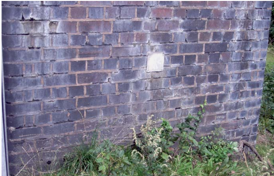
Plate 11: Detail of brickwork showing failing re-pointing
