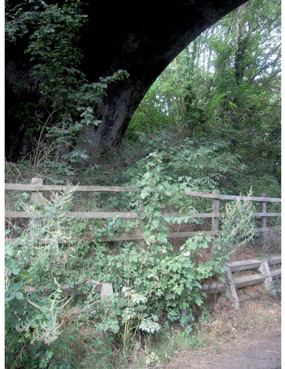
Plate 18: Detail of concrete retaining wall under the western arch of the viaduct
