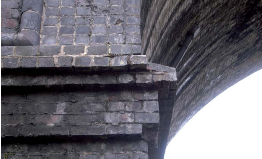
Plate 4: Detail of damaged stepped brickwork on north facing elevation
