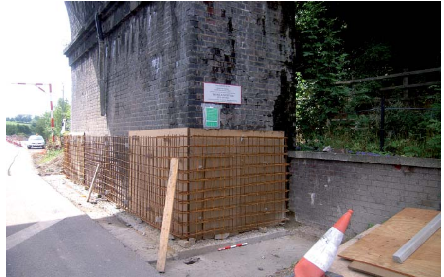
Plate 13: View of pier following removal of crash barrier and prior to construction of concrete barrier replacement
