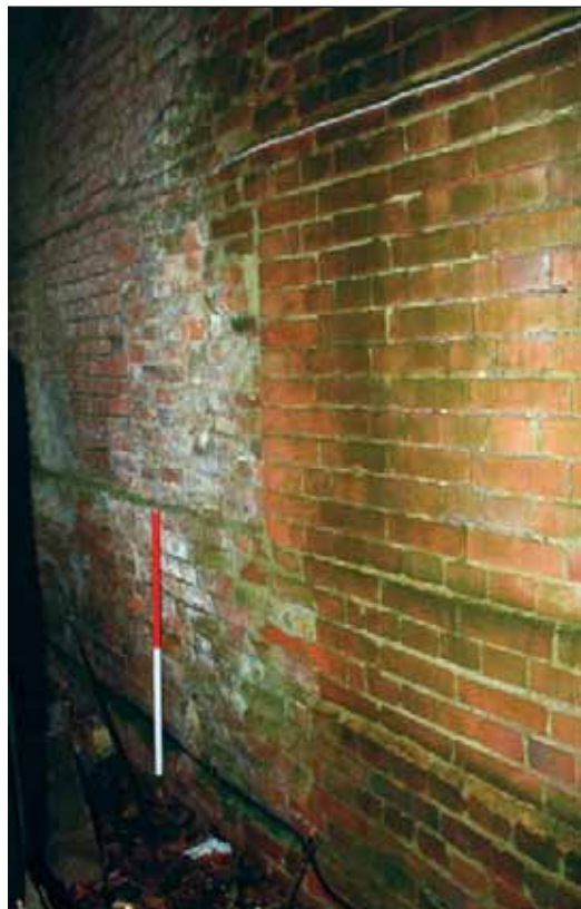
Plate 9: Detail of blocked up window and repair to brickwork on north-facing elevation
