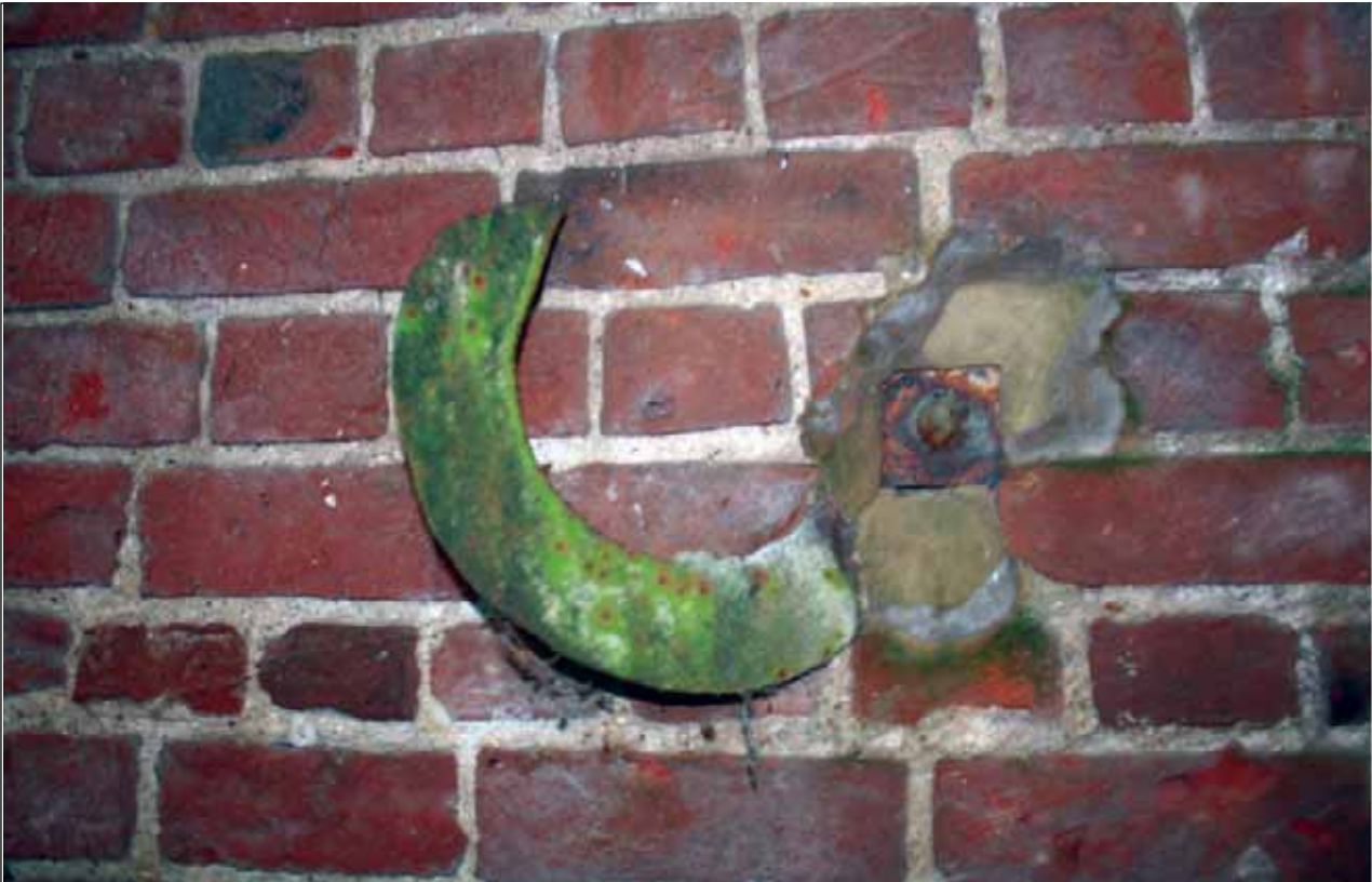
Plate 10: Iron structural tie on north-facing elevation
