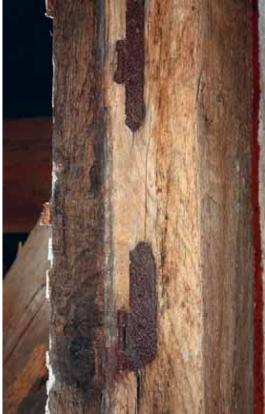
Plate 74: Remains of "H" hinges from doorway in roof space 1
