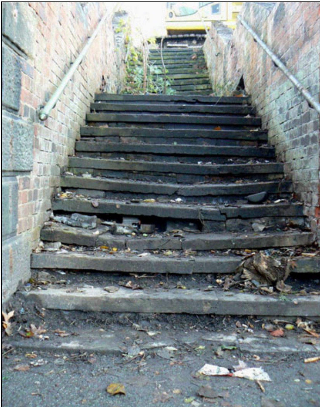
Plate 5: The Lowry Steps from Aspin Lane immediately prior to the repair works in 2013
