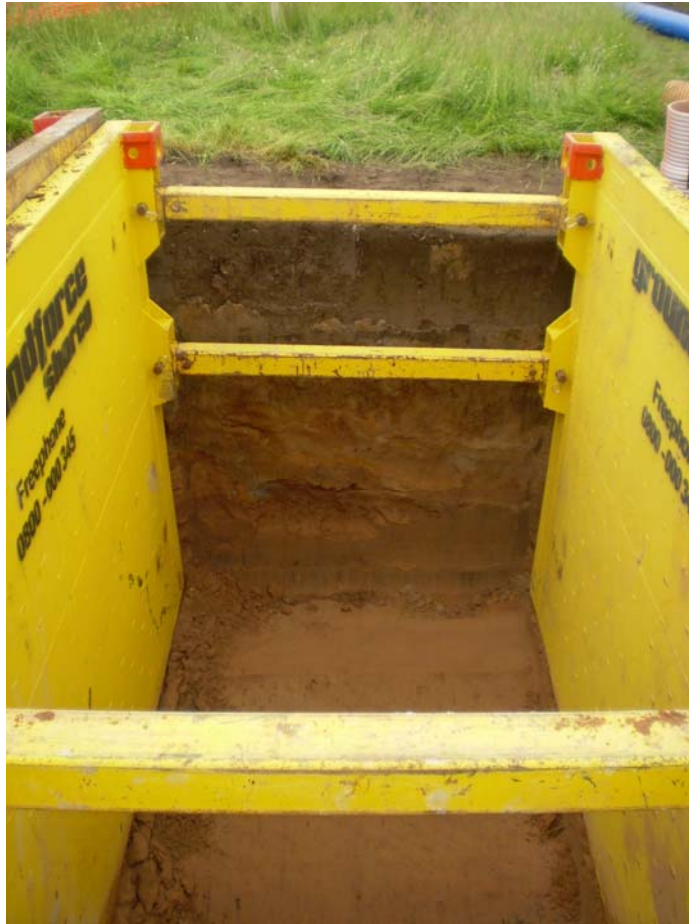
Plate 3: (Field 23) Section of directional drilling pit 23A showing deep alluvial deposit sealed by subsoil and topsoil
