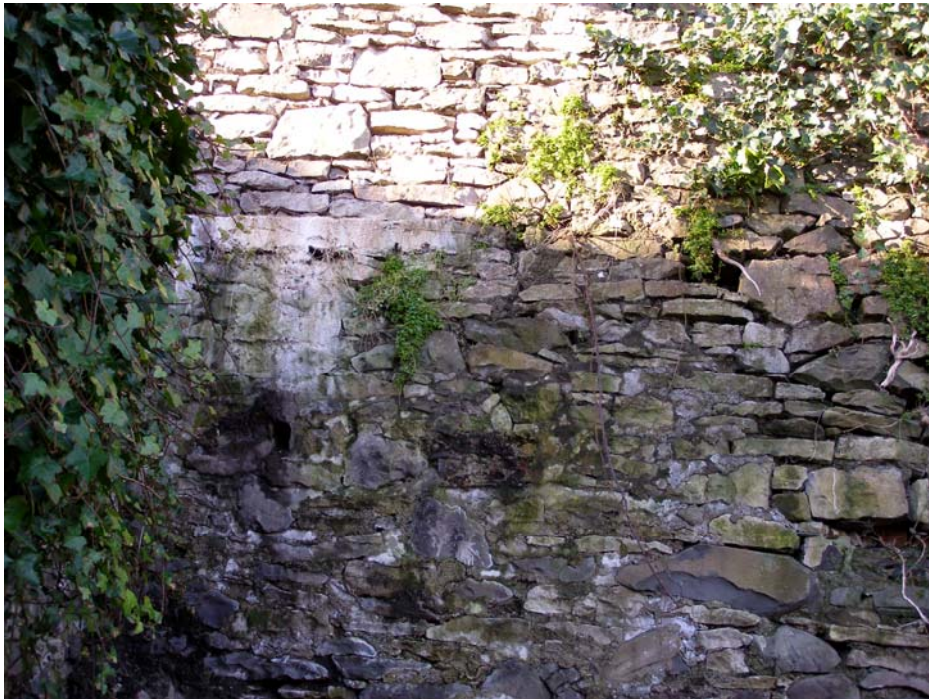
Plate 16: East-facing elevation of boundary wall, southern end showing the join between the earlier and modern wall.
