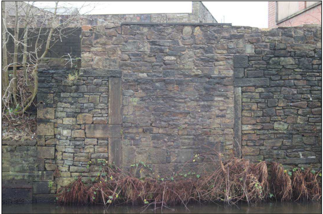
Plate 20: Blocked loading wharf entrance in canal wall
