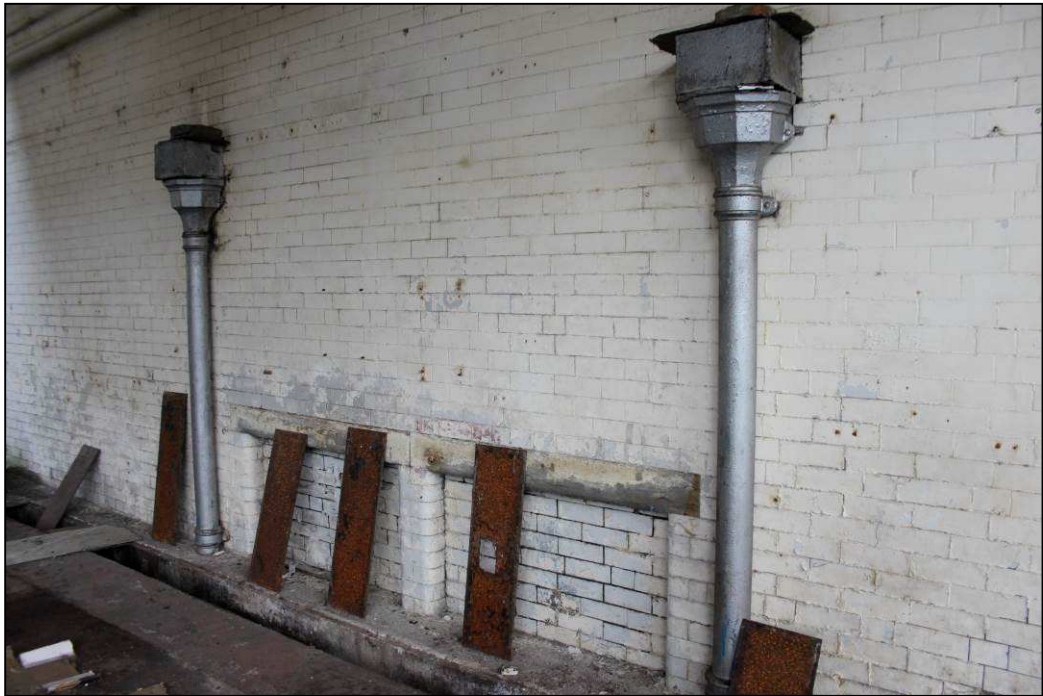
Plate 57: Blocked doorways to yard and internal downpipe hoppers
