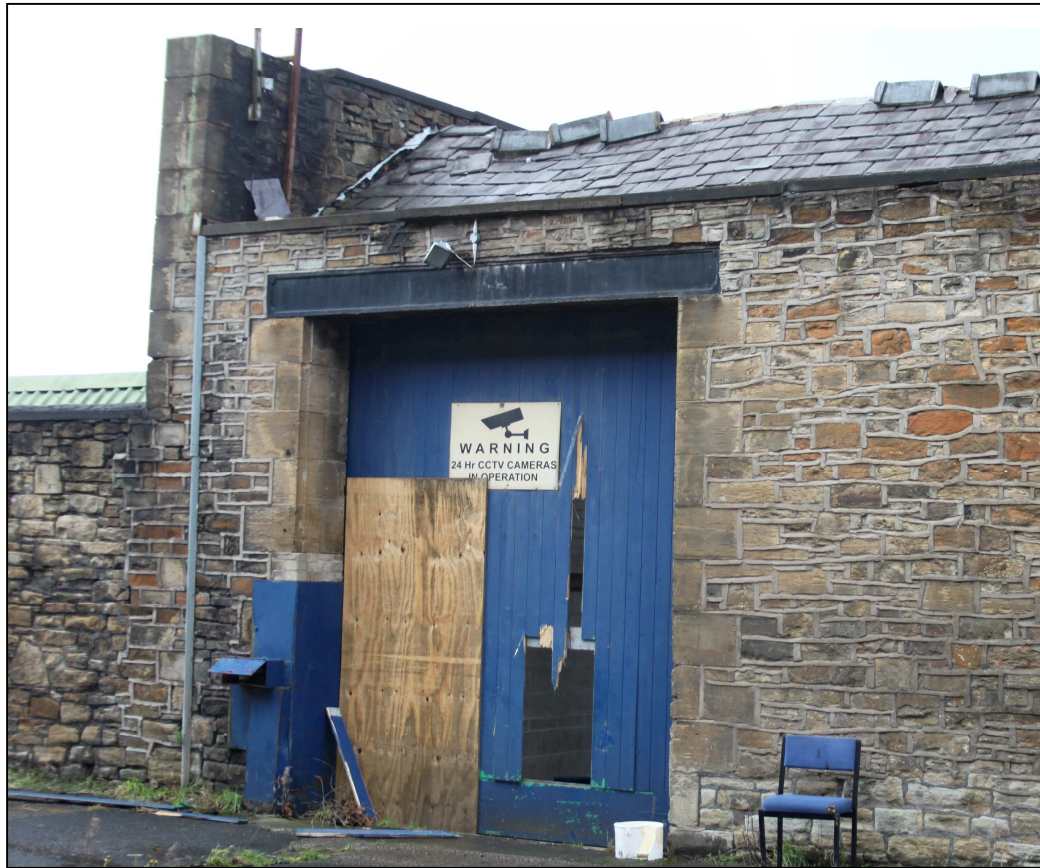
Plate 53: Western loading door in Unit 3
