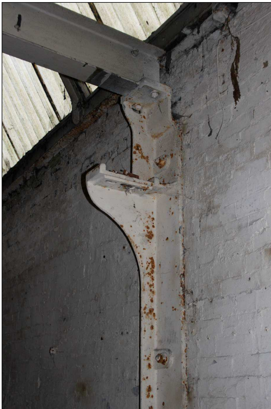
Plate 35: Cast-iron pillar for line shaft bearing, Unit 5
