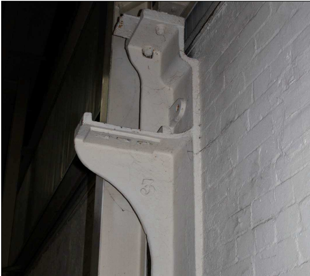
Plate 39: Cast-iron bearing support, Unit 6
