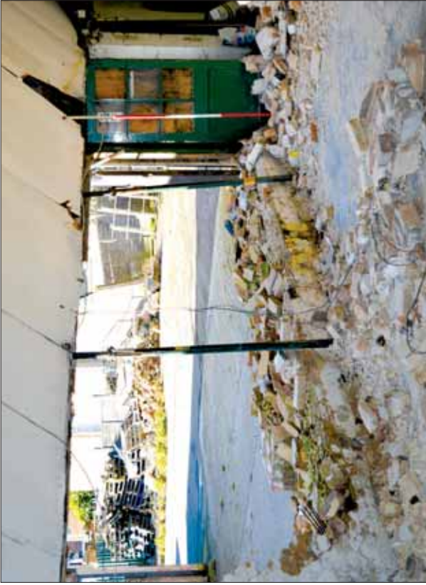
Plate 14: Collapsed southern wall to Room 1, from north-east
