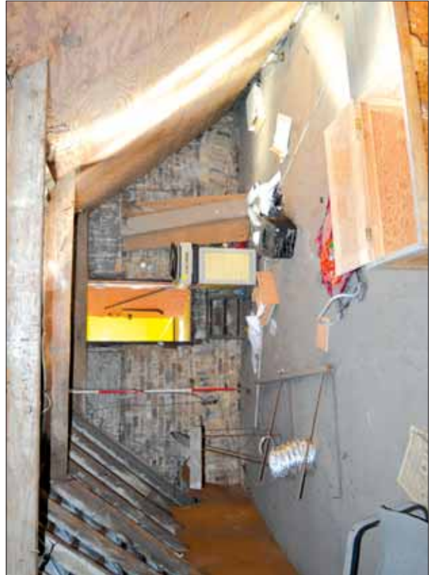
Plate 39: Detail of west wall to Room 8 showing doorway and relieving arch, from east
