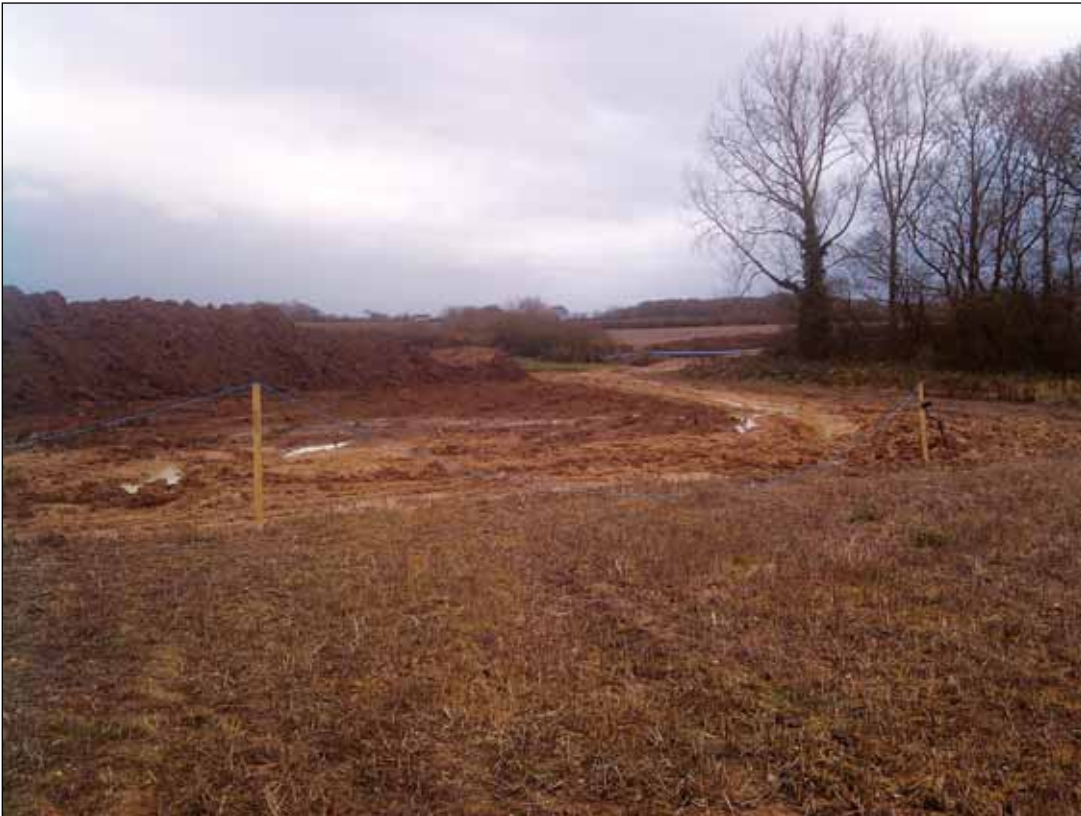
Plate 3: Chainage 850m, facing east - potential location of Lower Farm after topsoil strip
