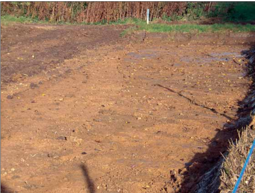
Plate 4: Chainage 1300m showing impact of adverse weather conditions on the site prior to the pipe trench cutting. Facing north-west
