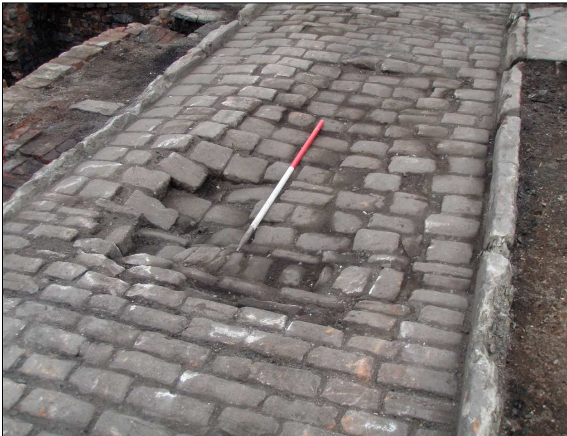
Plate 12: Localised collapse in the road surface, looking north
