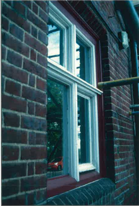
Plate 5: Window to be removed, front elevation
