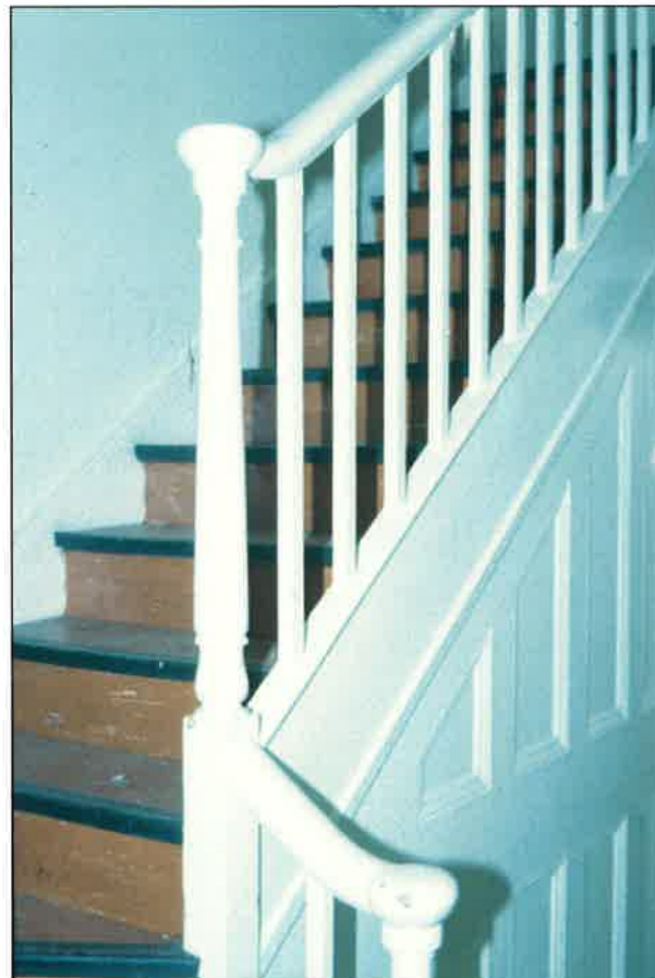
Plate 11: First floor staircase, detailing square balusters, rounded handrail, turned newel post and button top
