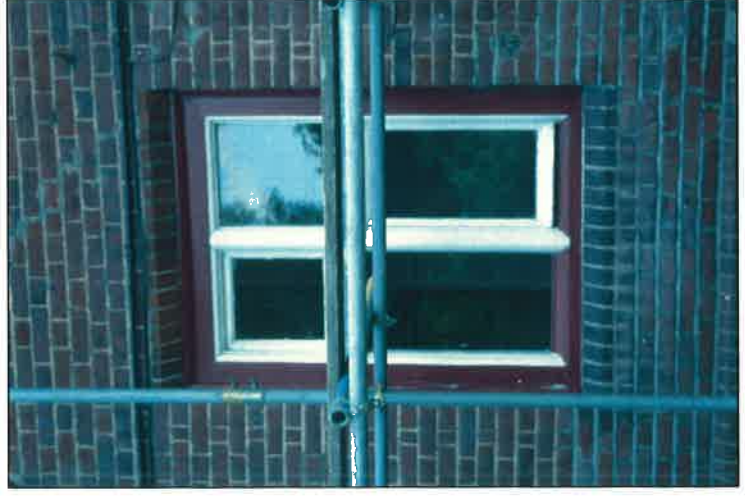
Plate 4: Window to be removed, front elevation
