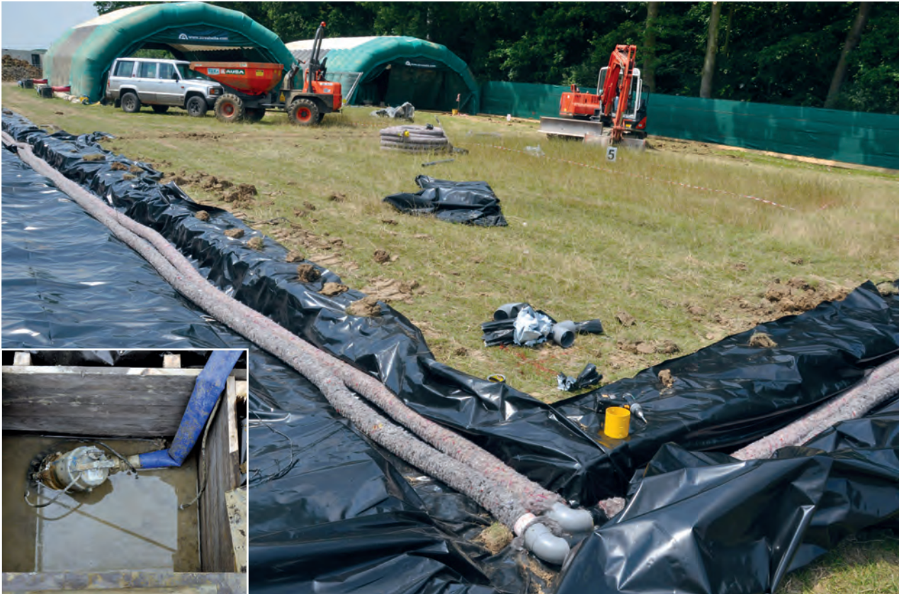
Fig. 2.10 Water management: a 'French drain' (main image) and pumps with sumps (inset) were among the strategies employed
