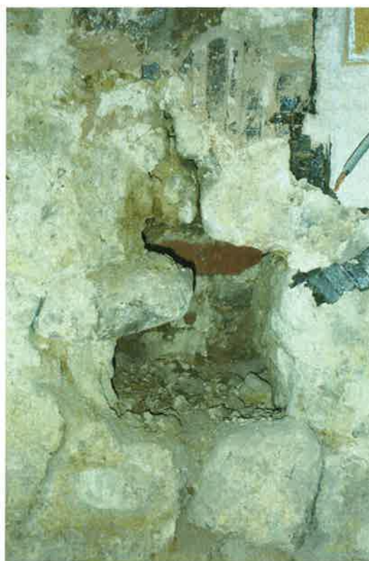
hole in wall
