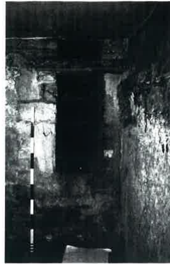
Plate 14: Thin window formed from previous wider opening in North wall of B/1.2
