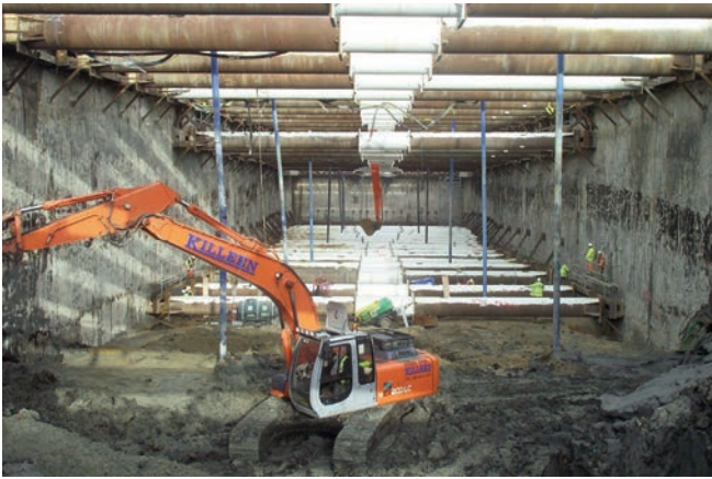
Plate 21 View of construction of cut and cover tunnel boring machine launch chamber, Swanscombe
